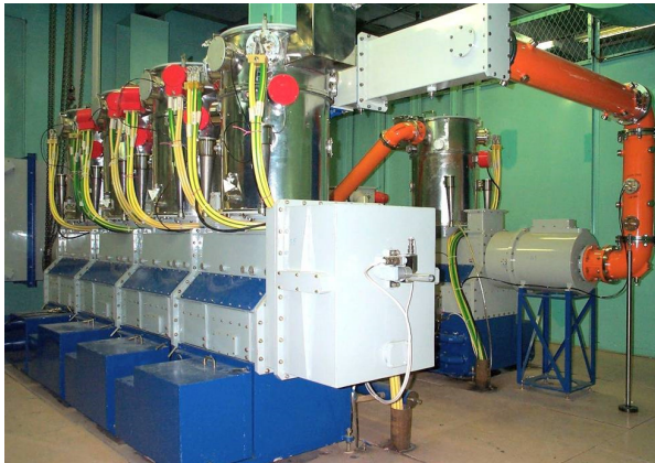
Figure 4. NovoFEL generators hall
