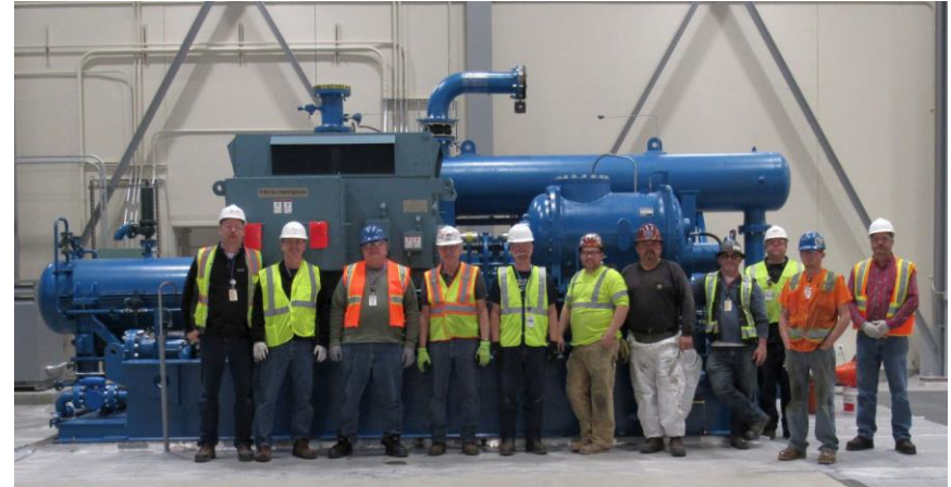
Warm Helium Compressor Installed
