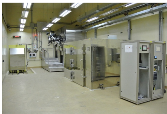
Figure 6: Cooling system and hot-cell.
