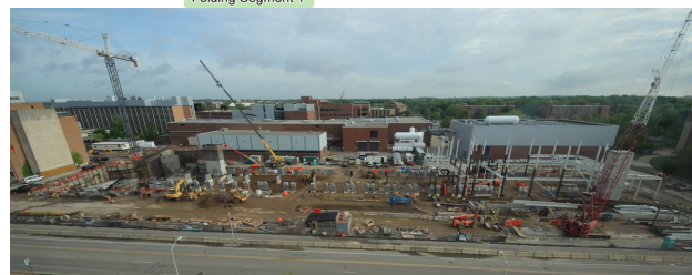
Figure 1: Layout of the FRIB driver accelerator, target and fragment separator (colored areas) and existing infrastructure (top); photograph showing FRIB civil construction (bottom).
