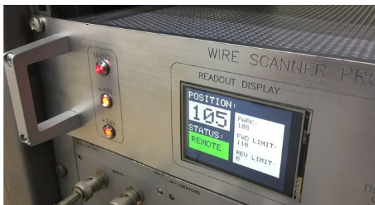
Figure 4: Motor control unit readout display.
