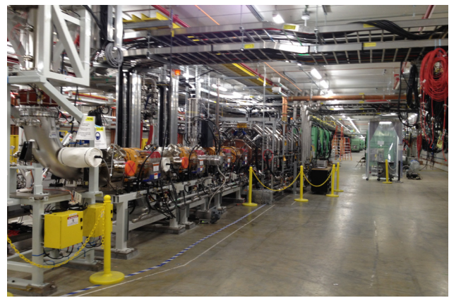
Figure 3: FRIB tunnel showing the lower LEBT and RFQ fully installed, and first QWR cryomodules aligned.
