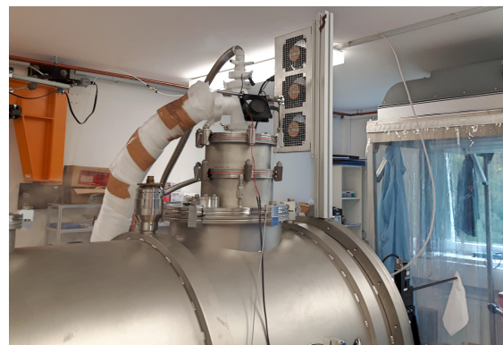
Figure 8: The cryomodule of Gun III during cooling with liquid helium.
