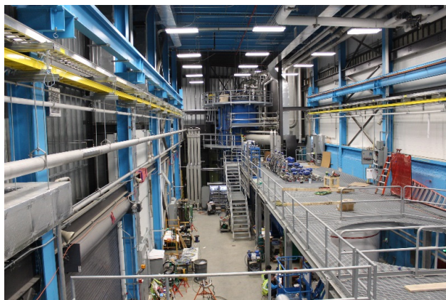
Figure 6: 4.5 K coldbox installed in the FRIB cryogenics building [9]. The Floating Pressure Process – Ganni Cycle [10] is implemented to provide efficient adaptation to the actual loads.
