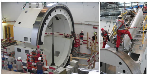
Figure 2: Installation phase, July 2015. Left : Front ring. Right : Installation of pre-assembled beamline girder.
