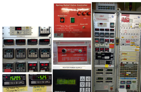
Figure 1: Old PID controller CN2001 for cold gas/liquid control in the TLS.
