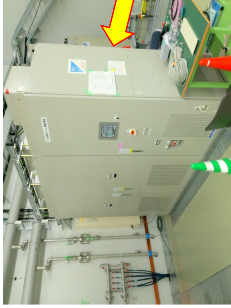
Power supply (60 Hz, 1 kV-299 A)
