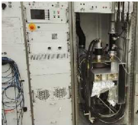
Figure 11: The SPS IOT system modified to 400 MHz and qualified to 60 kW (Courtesy E. Montesinos).
