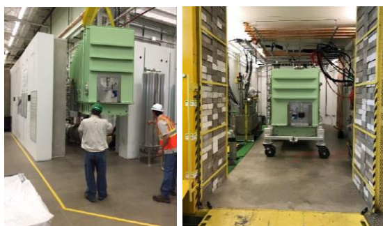
Figure 19: FRIB cryomodule bunker test systems. Left ReA6 bunker, right SRF Highbay bunker.
