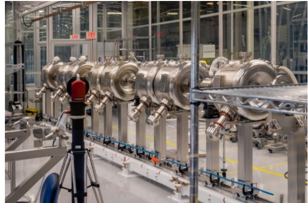
Figure 4: Eight 325 MHz couplers are installed to cryomodule string.
