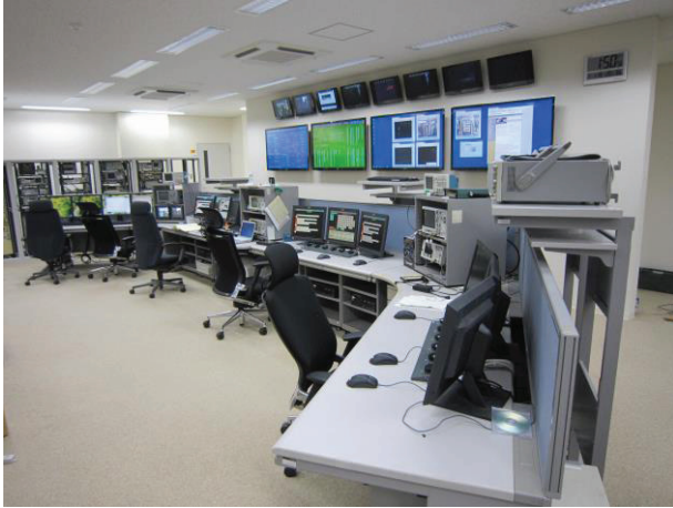
Figure 6: Control room after reform.
