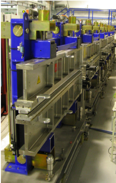
Figure 2 : Photo of the SPARC undulator chain during installation.
