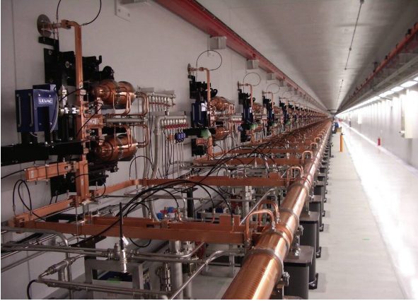
Figure 3: Photograph of the installed C-band accelerator in the tunnel.
