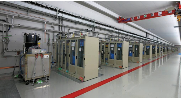
Figure 4: Photograph of the klystrons, the modulators and the control cabinets, placed alternately at every 4 m unit length, in the klystron gallery.
