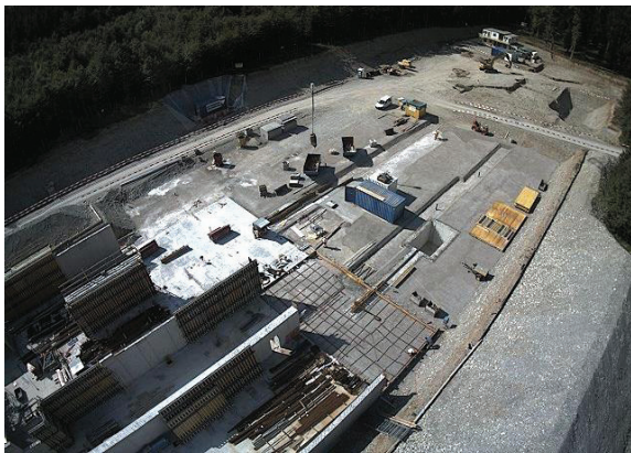
Figure 5: Picture of the SwissFEL construction site with the Aramis beam dump groove clearly visible.
