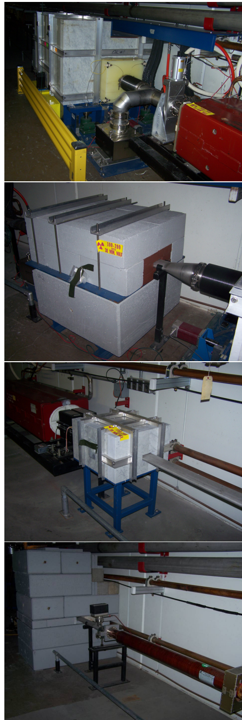
Figure 4: Examples of installed collimators: 20-Ton Secondary, steel and concrete mask (STCM), steel and marble mask (STMM) and the concrete wall are shown.
