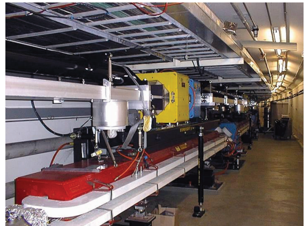
Figure 1: PEP-II tunnel with LER above the HER.
