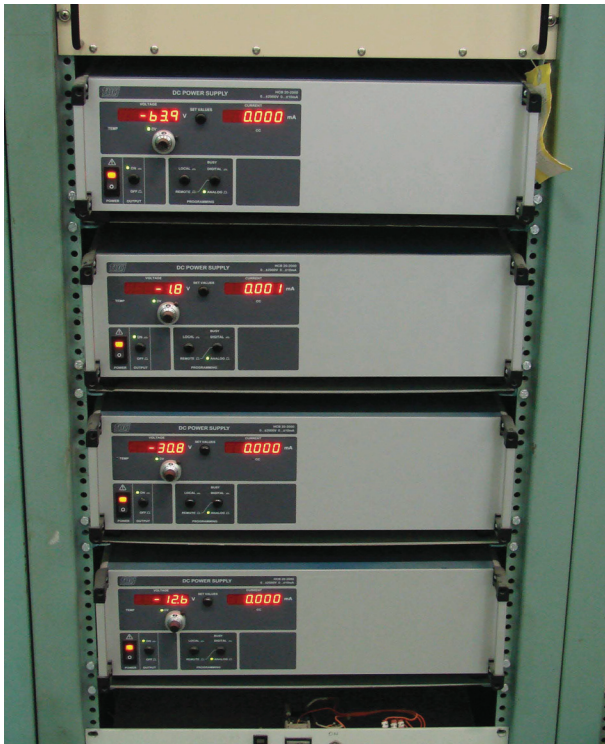
Figure 1: Bipolar power supplies block with continuous zero crossing capability for an electrostatic deflection system
