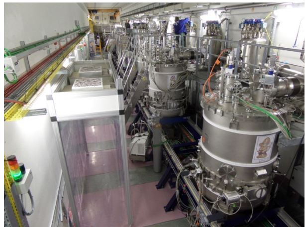
Figure 5: Low \beta (up) and high \beta (down) cryomodules installed in the linac tunnel (July 2015).
