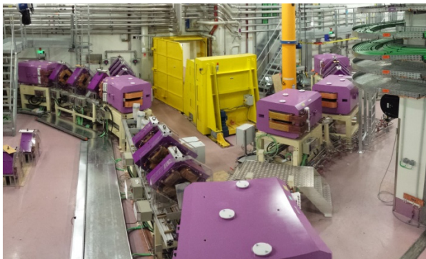
Figure 7: HEBT installation in the SPIRAL 2 building.
