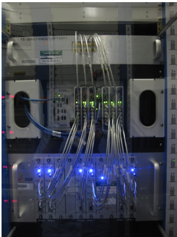
Figure 5: The new BPM electronics for the SNS MEBT in the rack.
