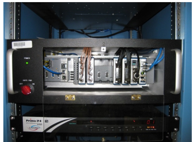
Figure 4: New BLM electronics chassis in the rack.
