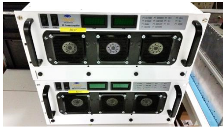
Figure 9: Two IBFB RF Power Amplifiers.
