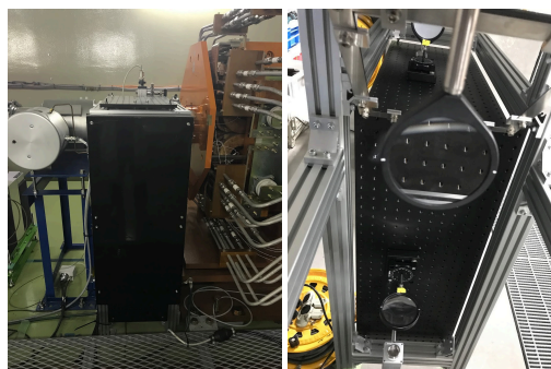
Figure 7: Optic system with frame installed in J-PARC neutrino beam line with front view (left) and inside with two lenses and 45° downward-mounted mirror (right).
