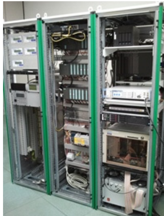
Figure 1: RFQ LCS Racks for Power Tests.
