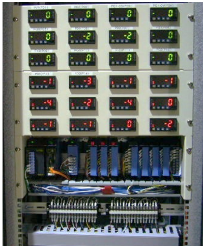
Figure 5: Digital panel meters and PLC of the interlock system for current fluctuations.
