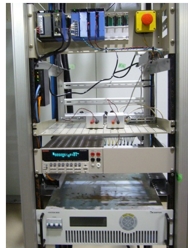
Figure 8: The power supply and PLC.
