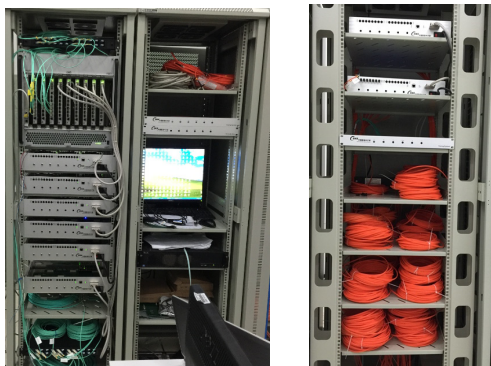
Figure 6: Photos of the central station and one of the local stations of the FPS.
