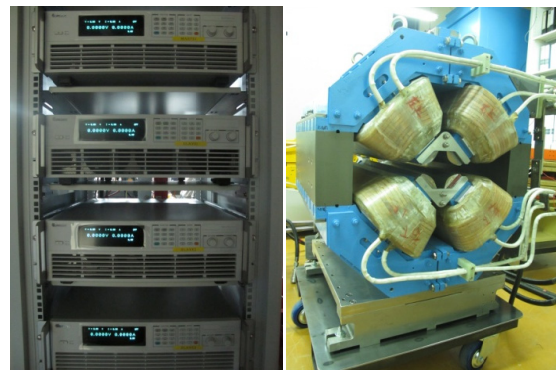
Figure 2: Chroma 62075H-30 power supply at laboratory
