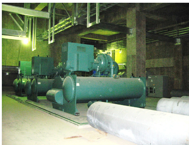
Figure 5: Three chillers installed in the Utility Building III.
