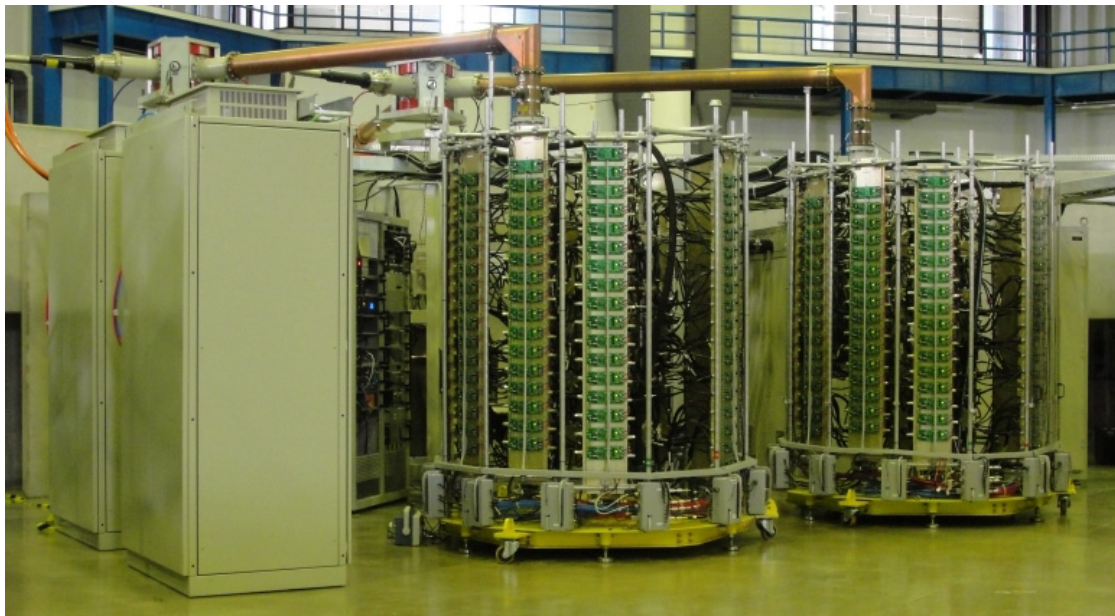
Figure 1: The two towers of the 50 kW solid state RF amplifiers operating in 476 MHz installed in the storage ring. From left to right the two 150 kVA DC power supplies, the racks of the low level RF and the two solid state amplifiers.
