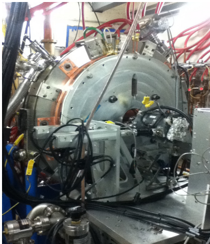
Figure 1: APEX cavity installed in BTF.
