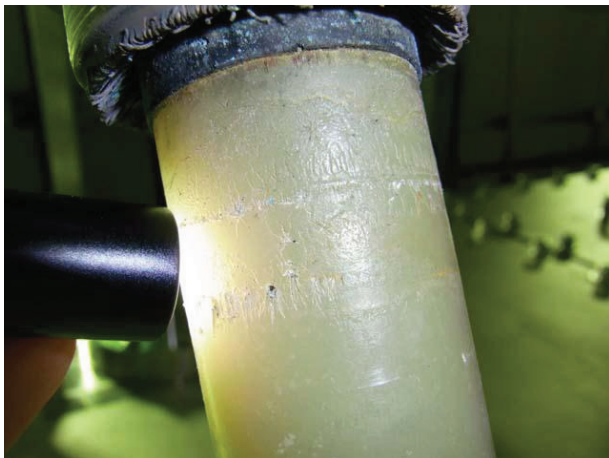
Figure 1: Scratches on the surface of polyethylene insulation layers.
