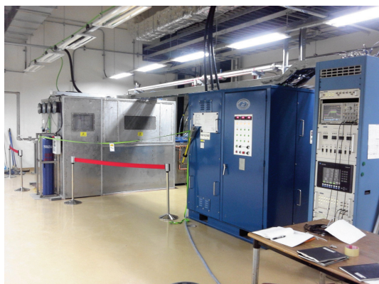
Figure 5: The modulator which was installed in the modulator room.
