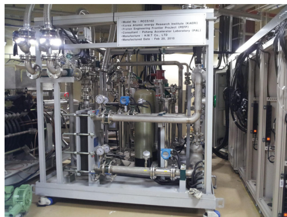
Figure 7: Resonant control cooling system installed in the klystron gallery.
