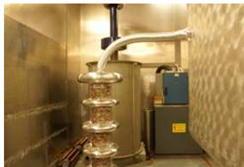
Figure 5: The Ohmlabs 250 kV (250 M \Omega ) dc HV divider specified for 10^{-4} precision, installed in the HV terminal of the electron cooler.
