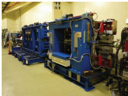
Figure 1: New elliptically polarizing undulator U#02-2 (near side) installed with the existing planar undulator U#02 (far side) in the long straight section.
