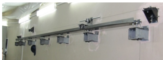
Figure 4: Rails along the wall to move the reflector laser system LMS- 100.
