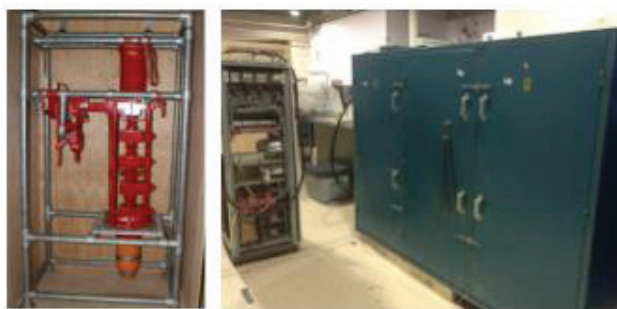
Figure 4: 1.3 GHz klystron and modulator system at CSU.
