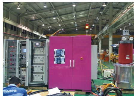
Figure 4: The first klystron modulator at the factory.
