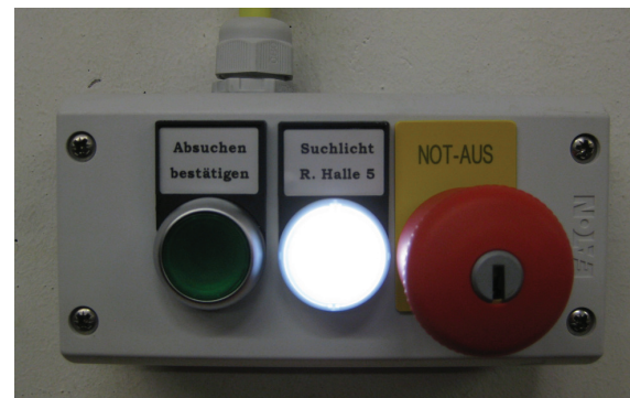
Figure 2: The box including the emergency shutdown button as well as a searching light and an always glowing light for orientation in the dark.
