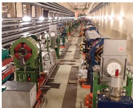
Figure 2: Magnets installed for new beam lines in the Tsukuba straight section.
