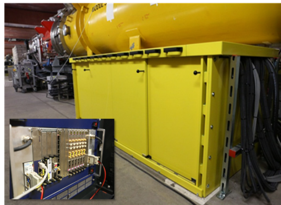
Figure 1: Installation of MicroTCA crates inside the FLASH tunnel underneath the accelerator module. The radiation shielding (yellow cabinet) protects the electronic rack inside. The insert shows the MicroTCA crate installed in this rack.
