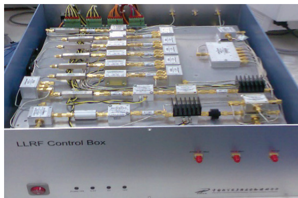
Figure 1: The first generation LLRF controller.
