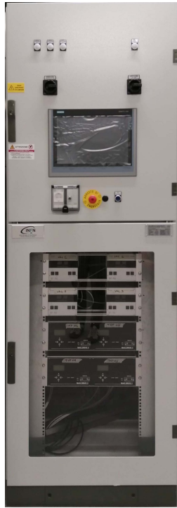
Figure 4: The new Vacuum Control Rack.
