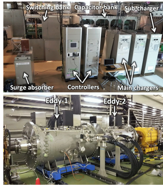
Figure 4: Photograph of PS for Eddy-1 (upper) and Eddy-1,2 installed in the MR (lower).
