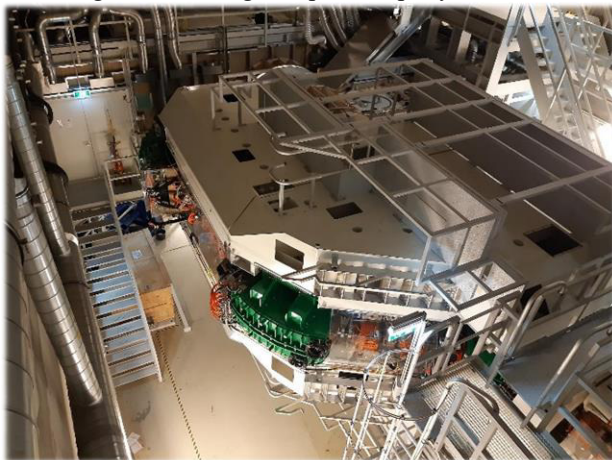
Figure 1: Bird view of the MedAustron gantry laying in the horizontal position. The gantry entrance is in the lower-right corner of the picture.
