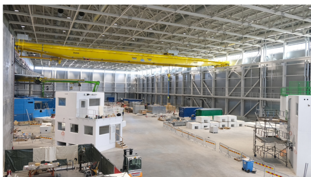
Figure 4: Photo of the South/East experimental hall showing ongoing construction of the ODIN and DREAM experiments (white) as well as the target bunker (blue) housing the choppers.
