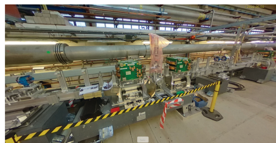
Figure 3: Current assembly status of the 2nd compression chicane (02.06.2022).
