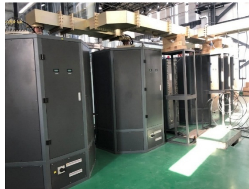
Figure 1: 650 MHz/150 kW SSA.
