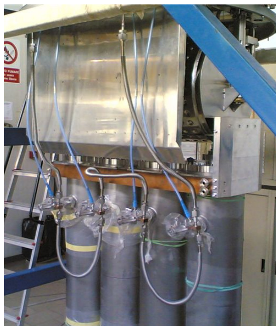
Figure 3: View of the flexible liquid Nitrogen line for rf coupler cooling and the Aluminum thermal shield.
