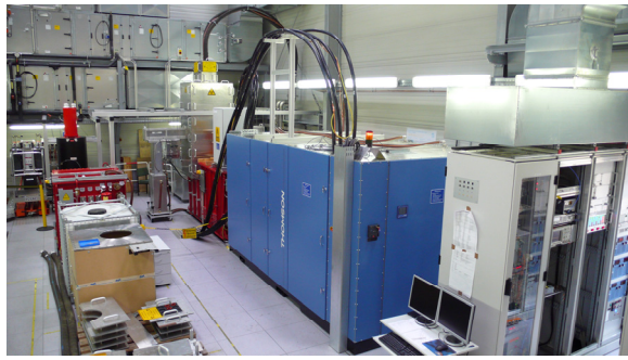
Figure 1: The new Modulator Test Hall.
