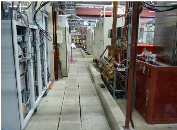
Figure 7: New RF station 3 with control racks.
