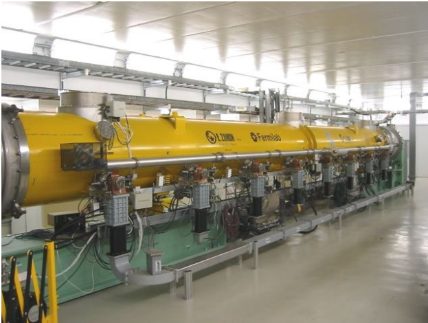
Figure 2: First installed cryomodule (CM1).
